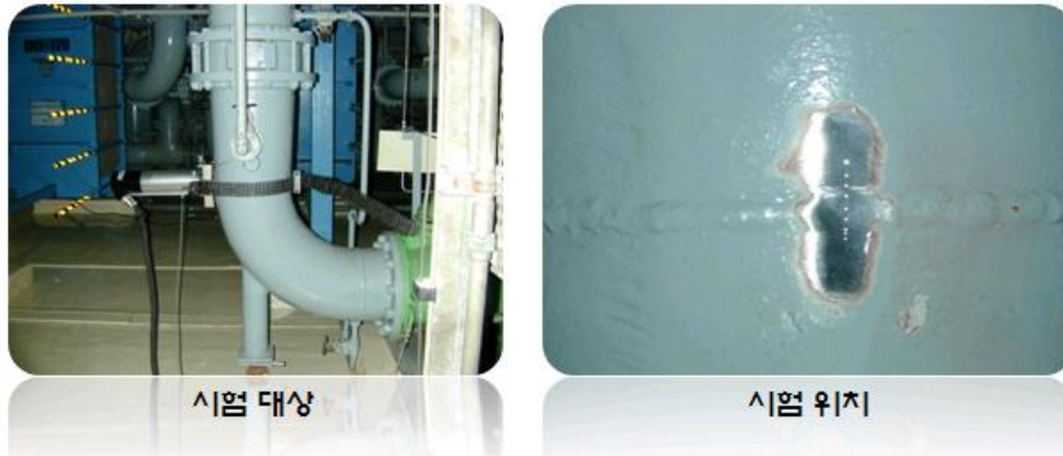
그림 19. Application case for main cooling water pipeline at nuclear power plant inspection using non-destructive indentation technique (at Kori in Korea)
