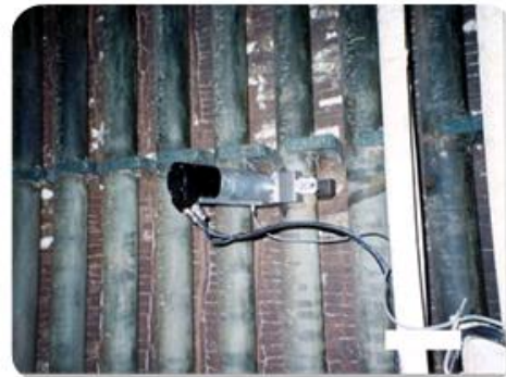
LG Caltex Oil (Vacuum heater tank pipe: A335 P5)
